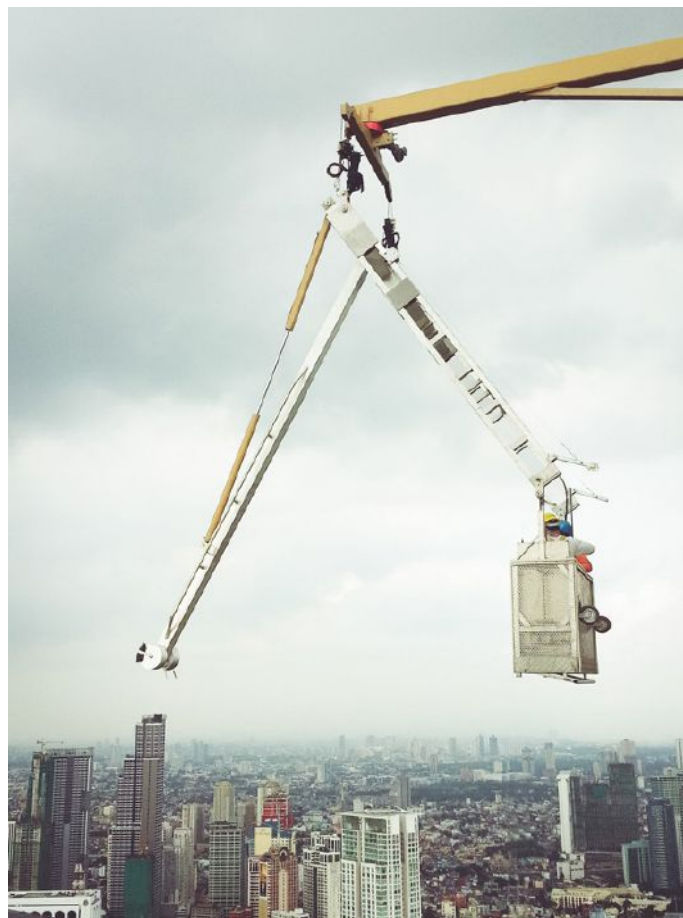
Machine with pantograph in the cradle to reach internal areas of the facade. Installed in Makati's yellow tower, in Makati, Philippines.
