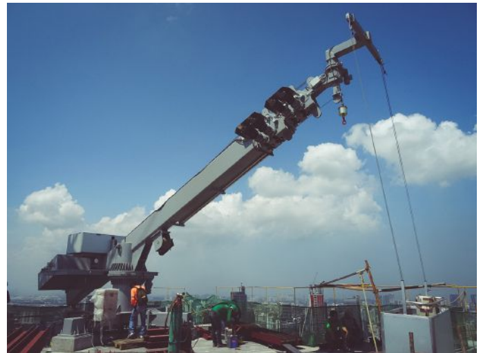
Trump Tower: a compact FBA S machine stationary and through slewing all facades can be reached confortably. Installed in Manila, Philippines.
